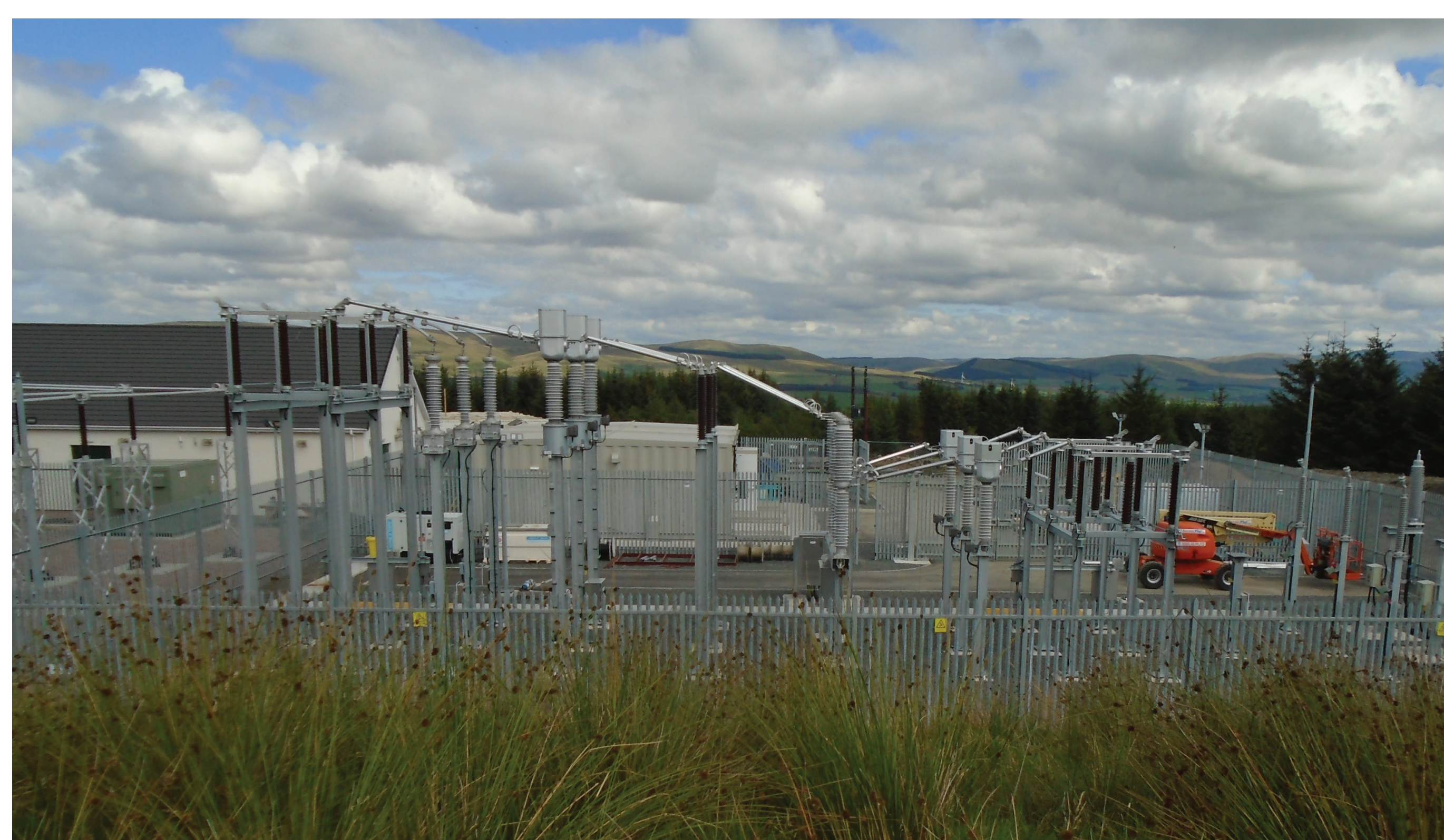
Typical circuit breaker compound
