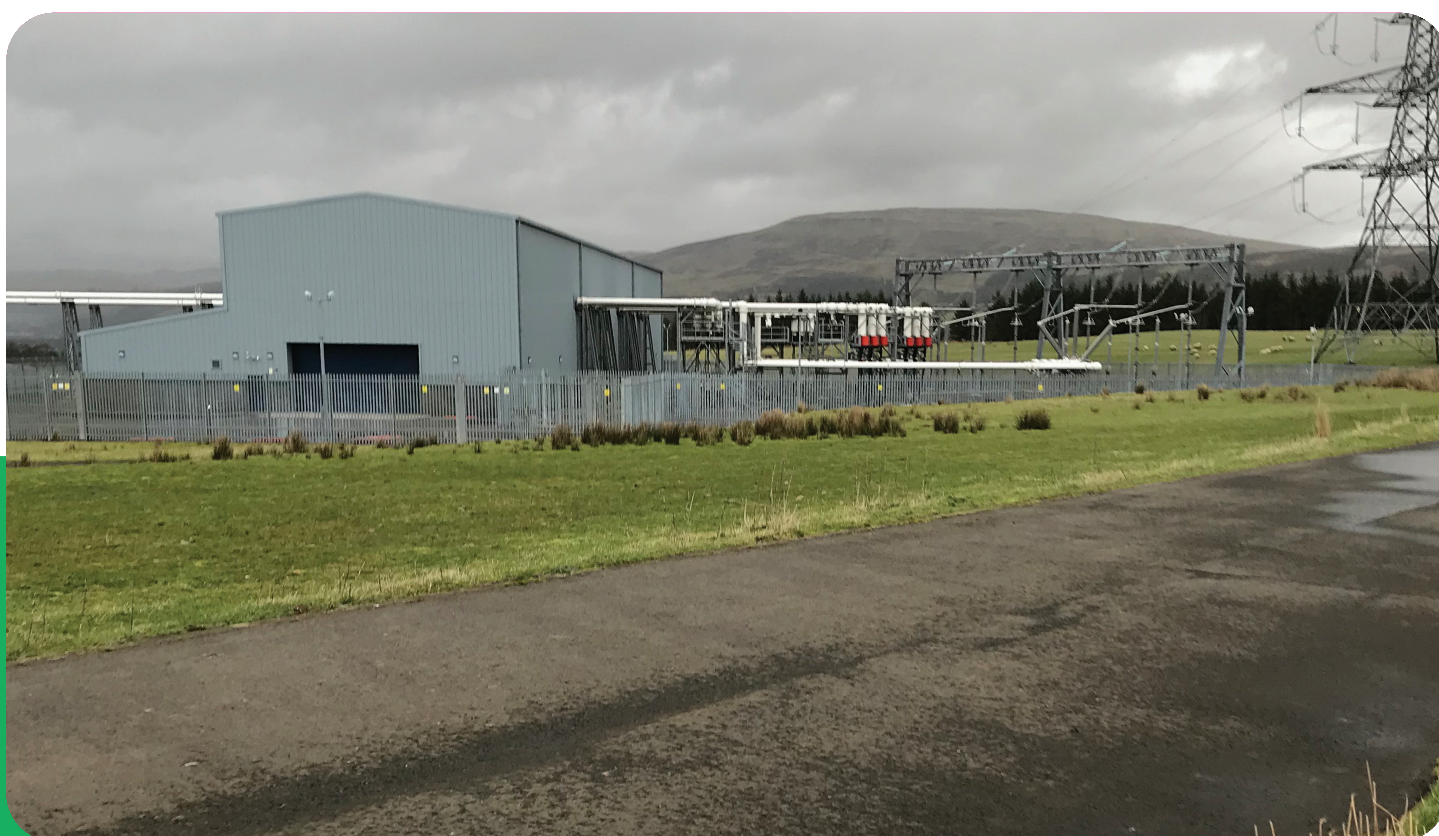
Hunterston East Substation
