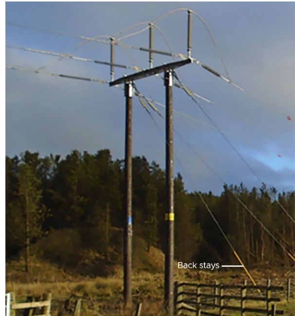
Photo 2: Typical H-Pole with Backstays
