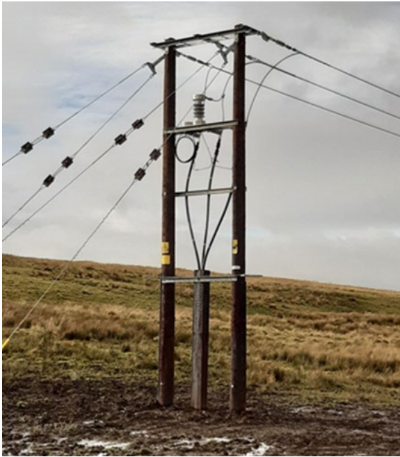
Photo 3: Typical Terminal Structure
