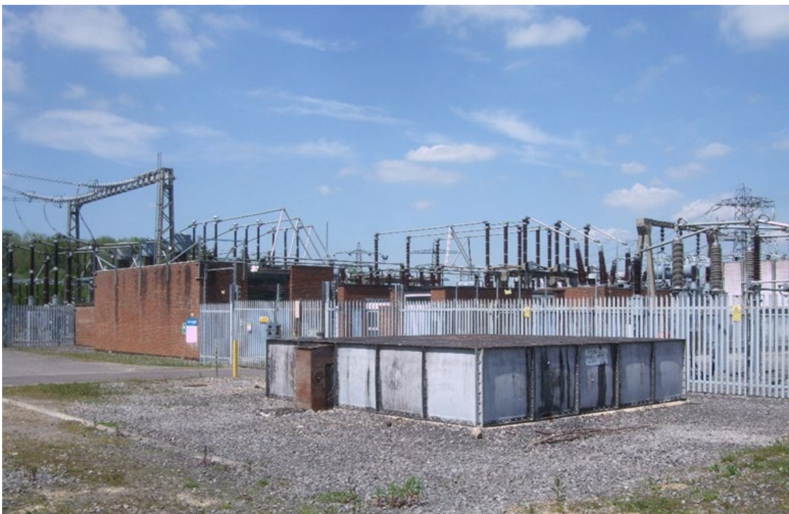
Typical 132 kV Substation
