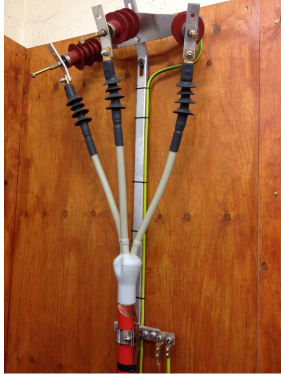
3-core overhead termination + earthing
