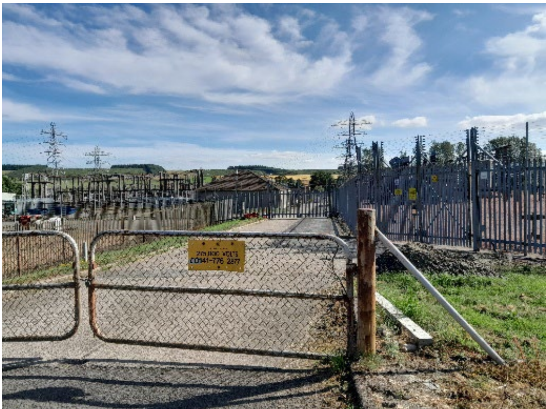
Image 3.1: Westfield Substation Access.
