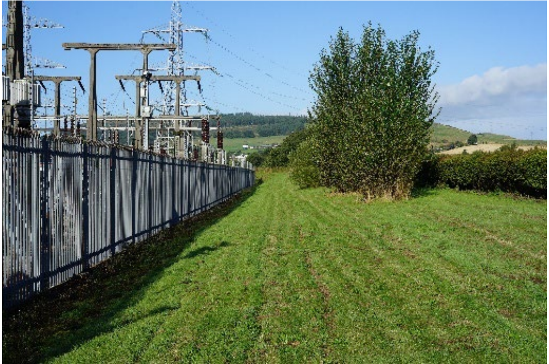
Image 3.4: Westfield Substation Northern Boundary Adjacent to B9097.
