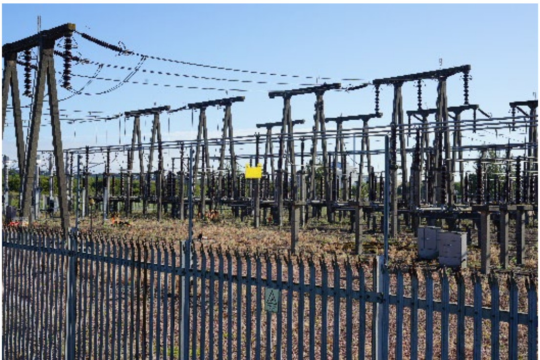
Image 3.3: Westfield Substation Existing Infrastructure.
