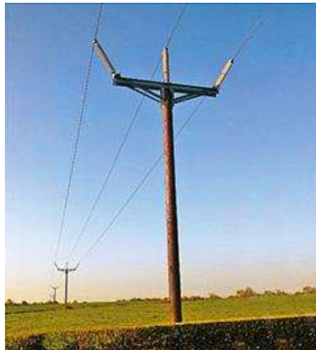
Figure 2.1: Typical Trident Wood Pole
