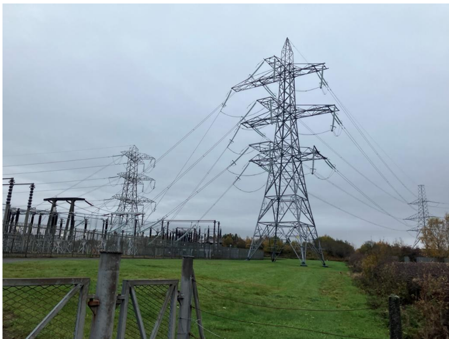
Photograph 9-50: View of the southern section of the Newarthill Substation. The works will be within the footprint of the existing substation.
