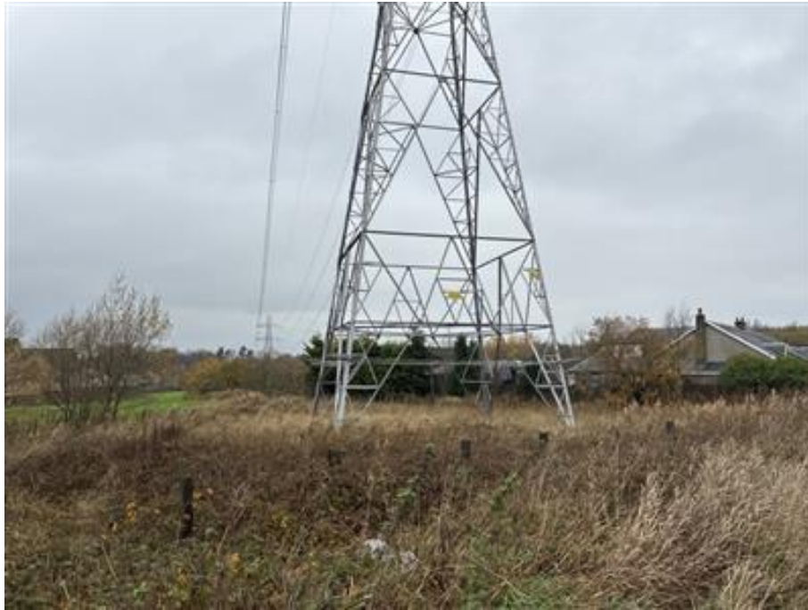
Photograph 9-17: View of Tower XX025 and bellmouth.
