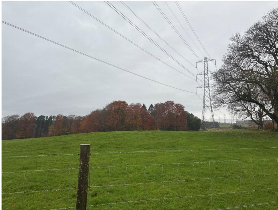
Photograph 9-23: Views of the XR overhead line as it passes through the former Allanton Parkland.
