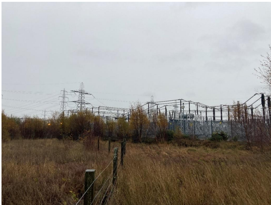
Photograph 9-38: View from the scheduled Doghillock Dun (SM6929) boundary looking west towards the existing Denny North substation.
