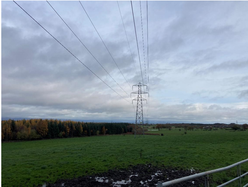
Photograph 9-30: Views northeast looking towards Tower CB027
