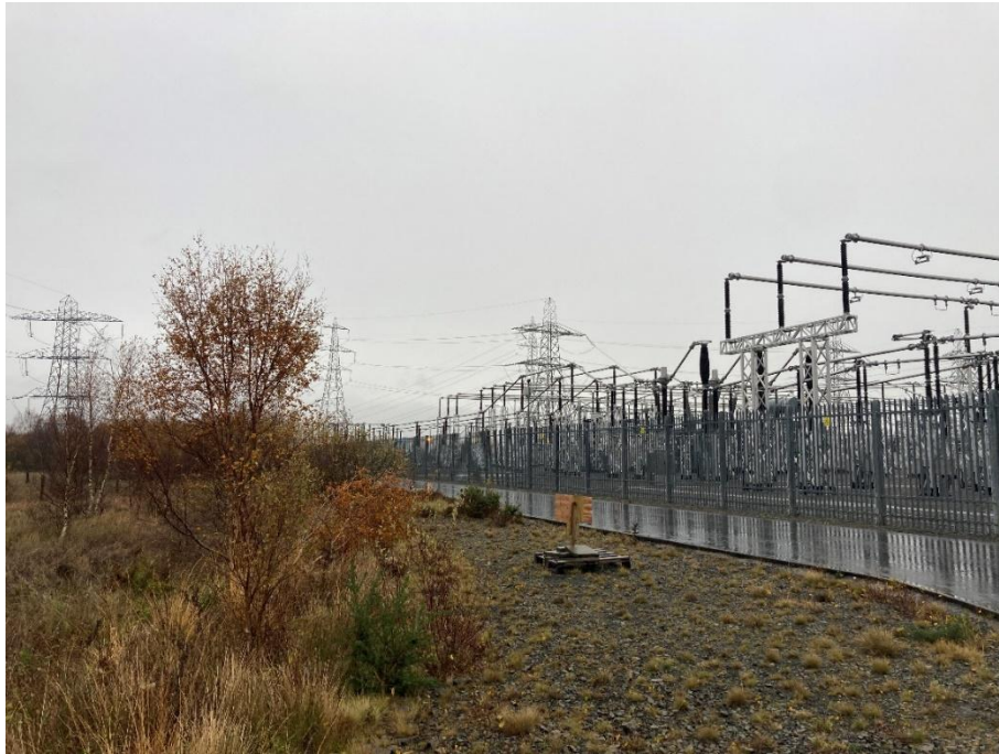
Photograph 9-33: View of the northwestern element of the existing Denny North substation.
