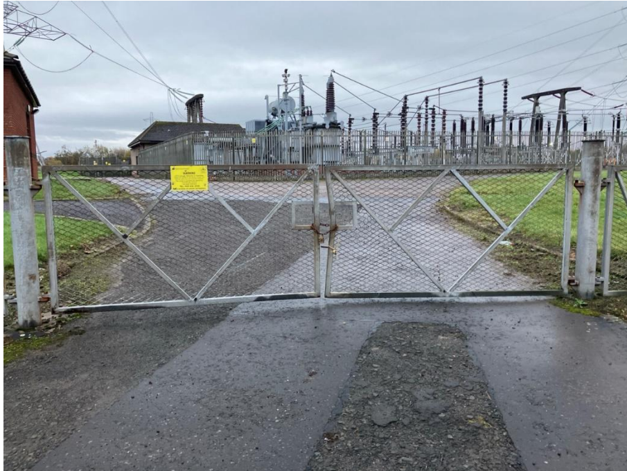
Photograph 9-49: Views of Newarthill Substation from the west.
