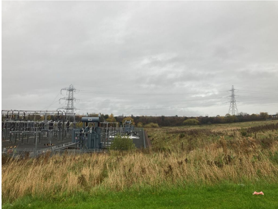
Photograph 9-51: Views of the eastern end of Wishaw Substation in the area of the works.
