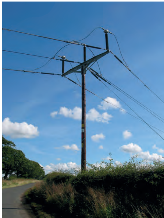
Trident single pole, vertical insulators
