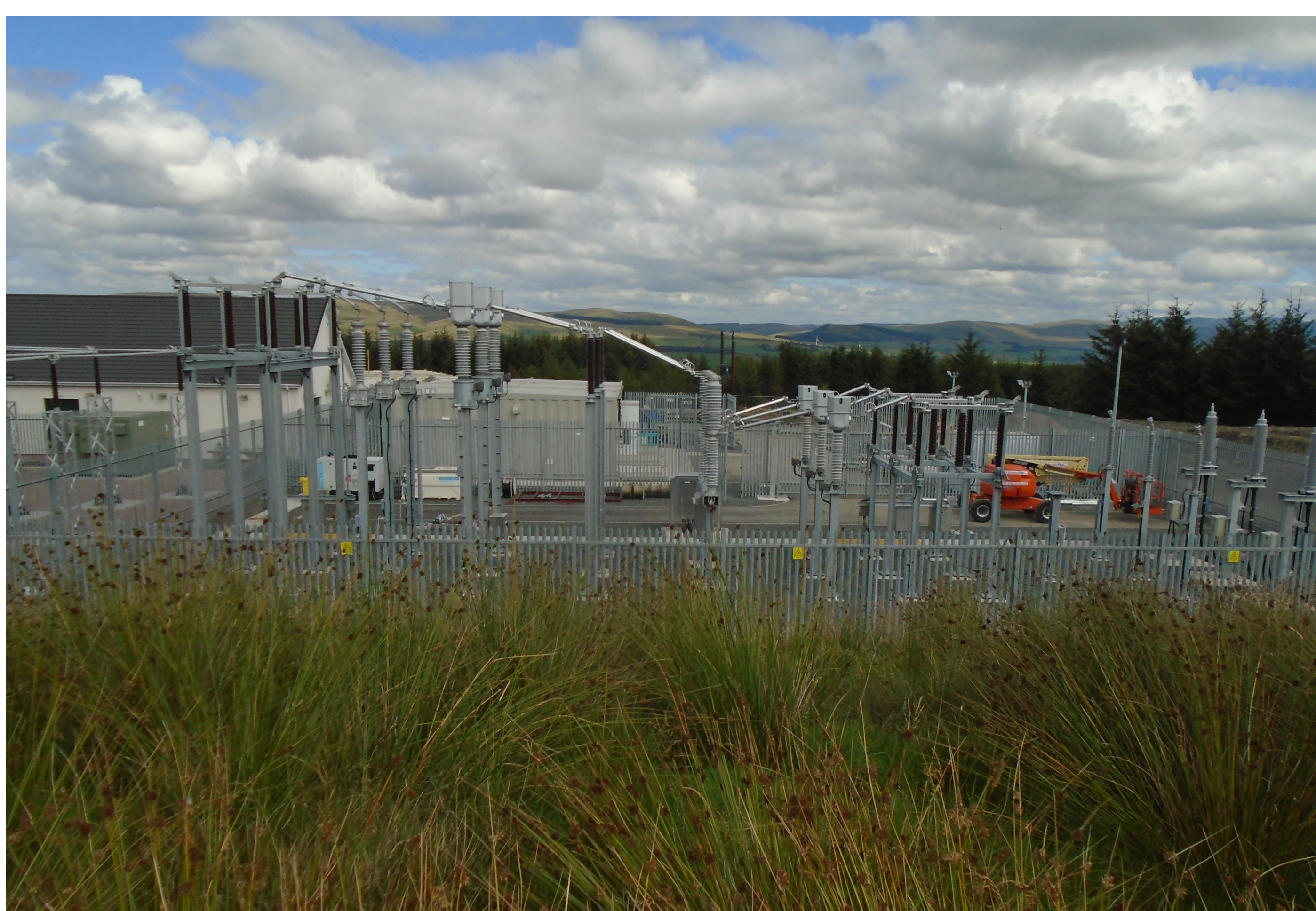
Typical circuit breaker compound
