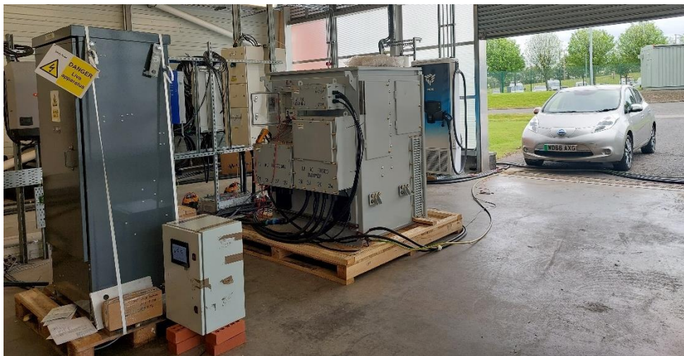
Figure 7 Network integration testing set up at PNDC
