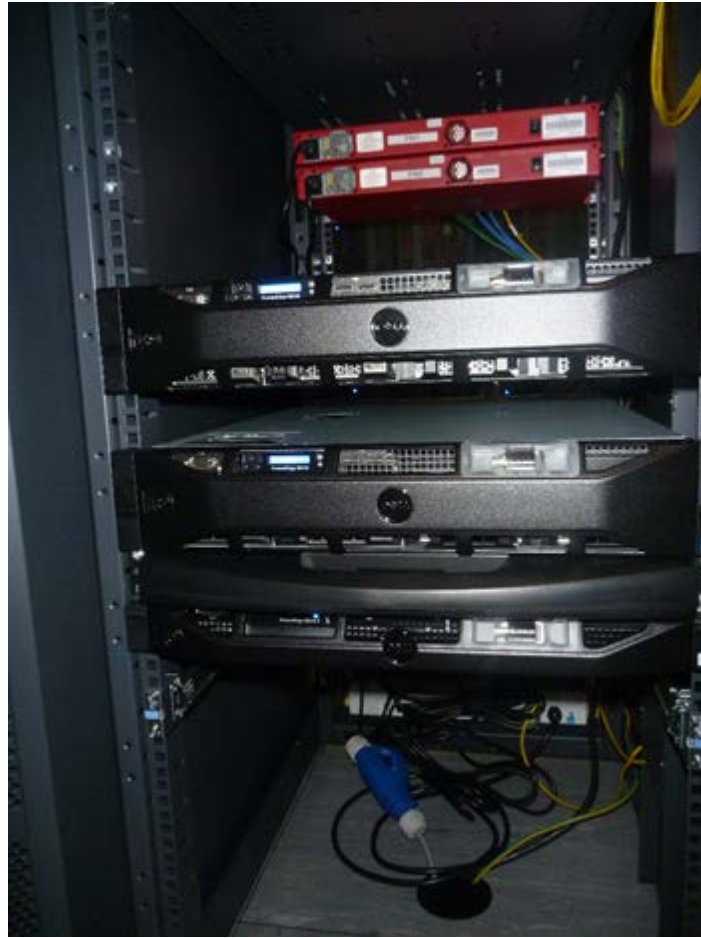
Figure 2 - Servers installed in the data centre
