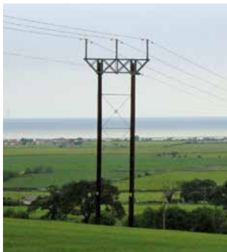
Heavy duty double wood poles – approx. 15m
