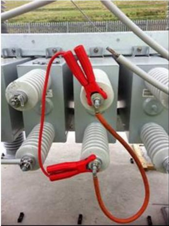
(Fig 7) Bolted Short- Circuiting Lead applied to Capacitor Unit.
