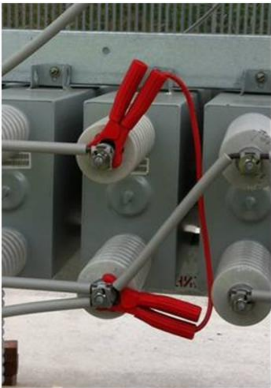
(Fig 6) Temporary Short- Circuiting Lead applied to Capacitor Unit before disconnecting capacitor unit.
