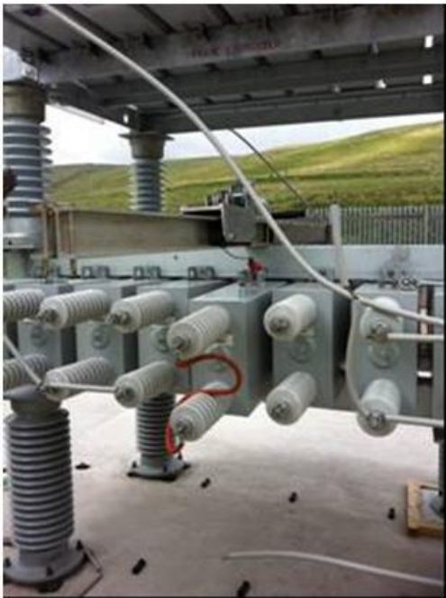
(Fig 8) Capacitor Unit can now be removed.
