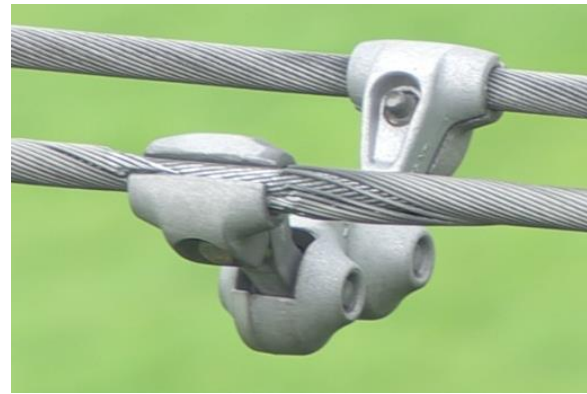
Conductor damage at span XJ088-089
