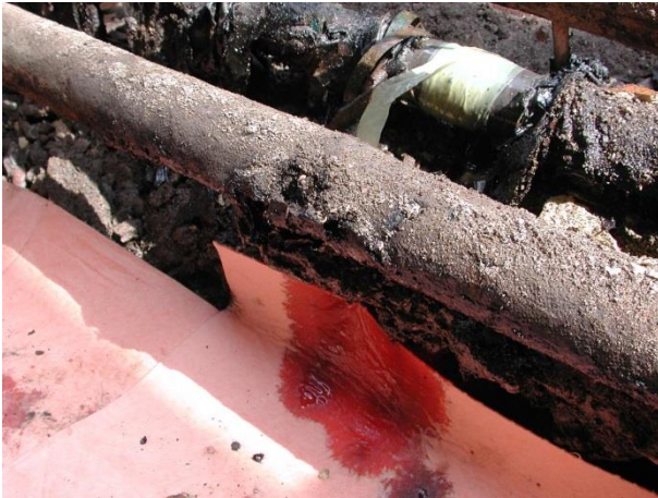
Figure 1: Damage [REDACTED] 2009 (Gorgie-Telford Road circuit)
