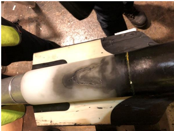
Figure 5: post-mortem termination inspection.
