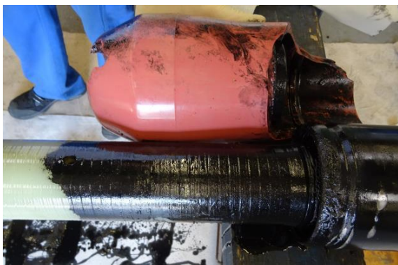
Figure 9: post-mortem termination inspection.
