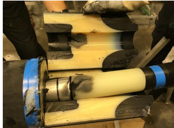
Figure 8: post-mortem termination inspection.
