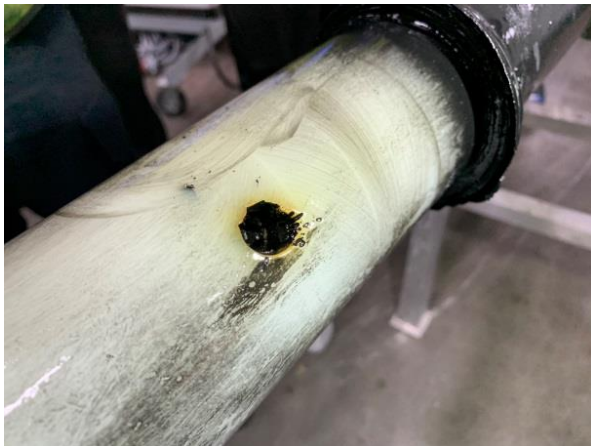
Figure 11: post-mortem termination inspection.
