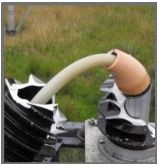
Figure 3 (Gretna): failure August 2016.
