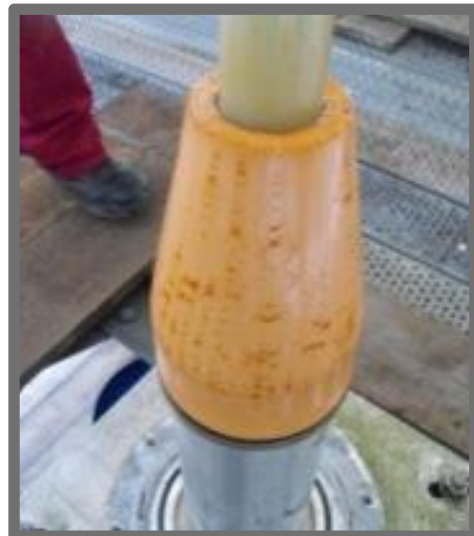
Figure 2 (Gretna): oil result failure April 16.
