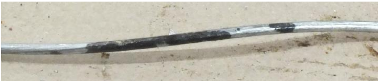
Figure 2: steel core strands exhibiting rusting after removing grease.
