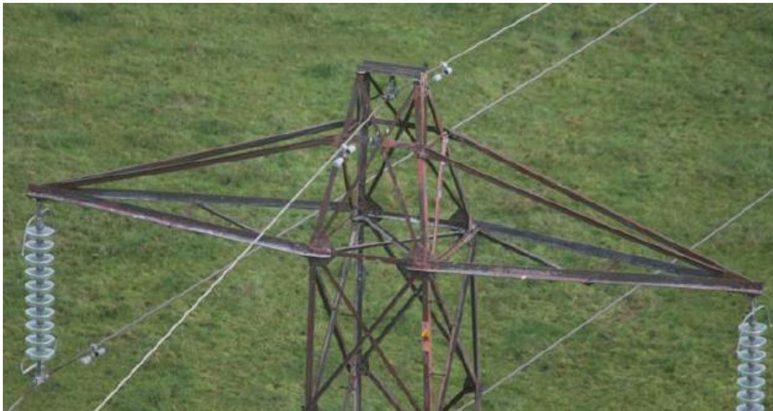
AY021 Tower: red prime visible and rusty steelwork.
