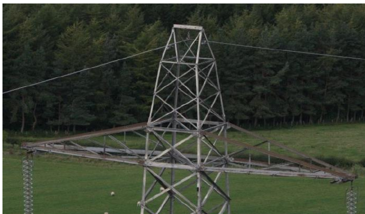
Figure 5: typical non-painted steelwork condition showing rust.
