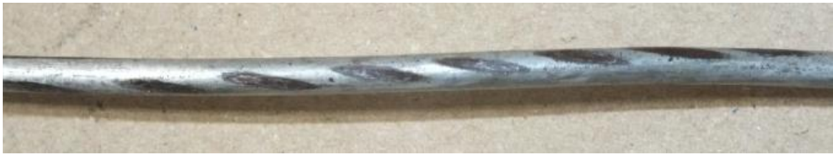
Figure 1: erosion of steel wires damaging zinc coating and exposing the steel bulk material.
