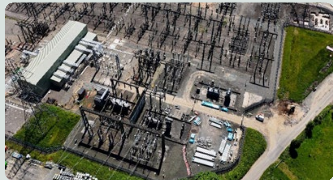
Bottom left: Picture of SF 6 free GIS in 132kV New Cumnock.
