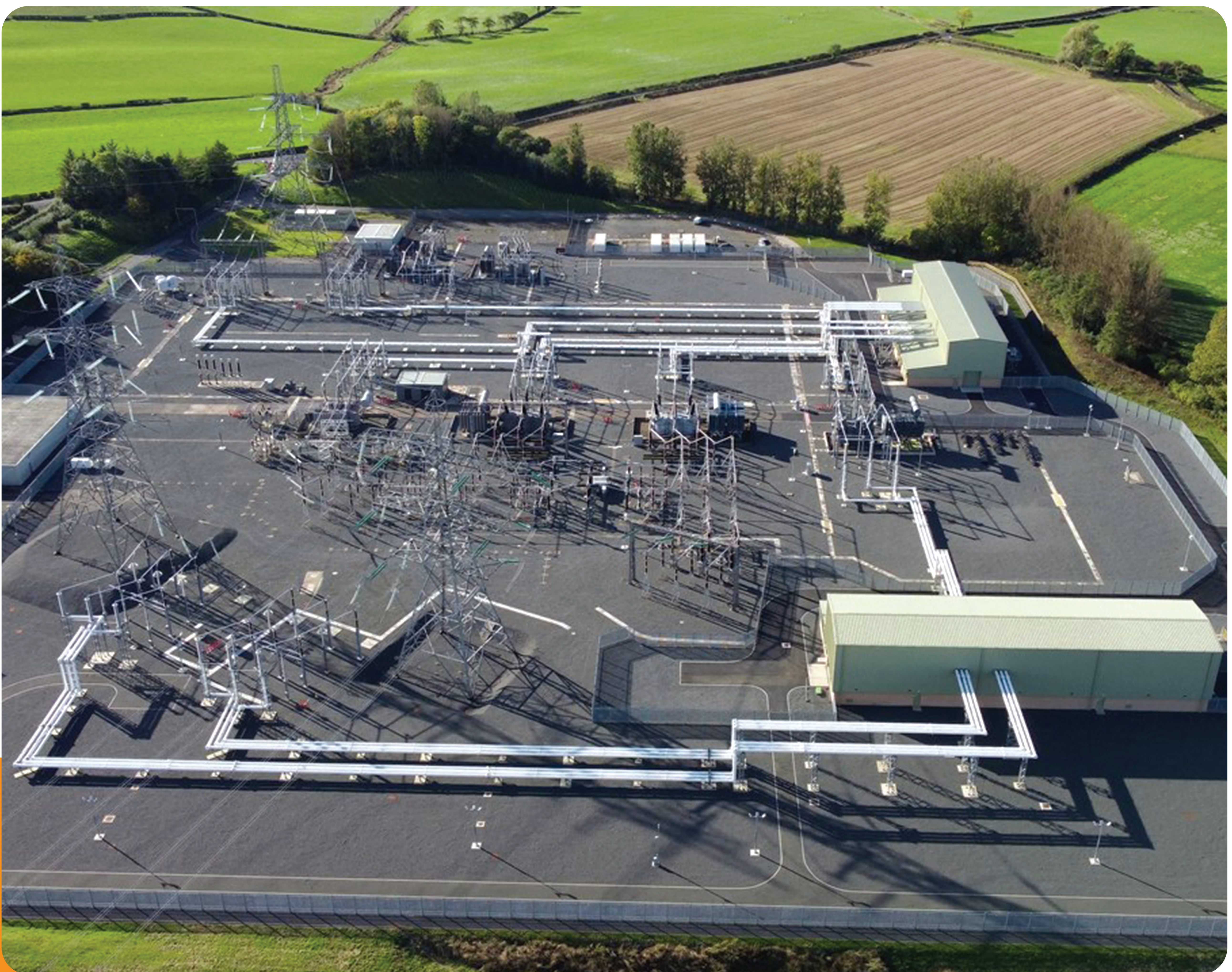
Figure: Example substation
