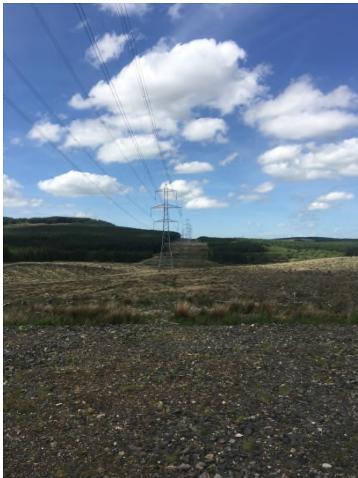
View of the recently installed 275kV WA Overhead Line between Coylton and New Cumnock substations
