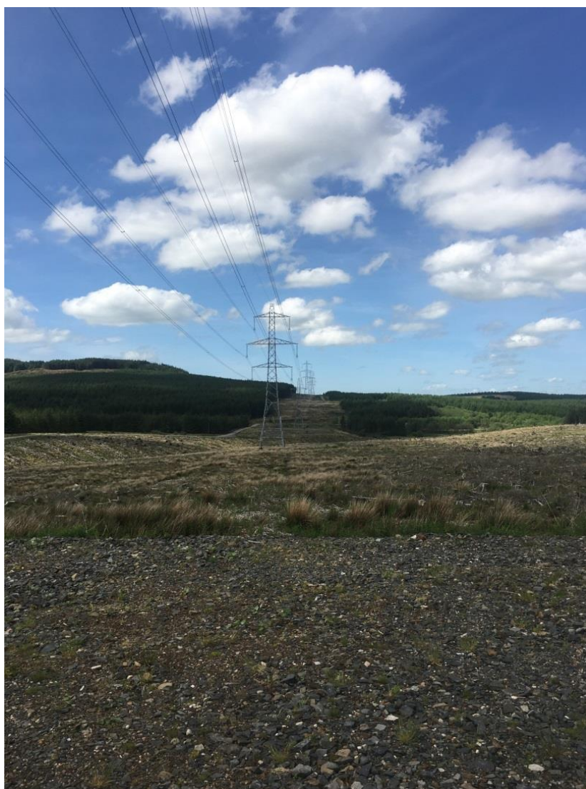
View of the 275kV WA Overhead Line between Coylton and New Cumnock substations
