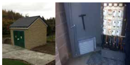
Figure 7 LV substation where the monitoring devices were installed
