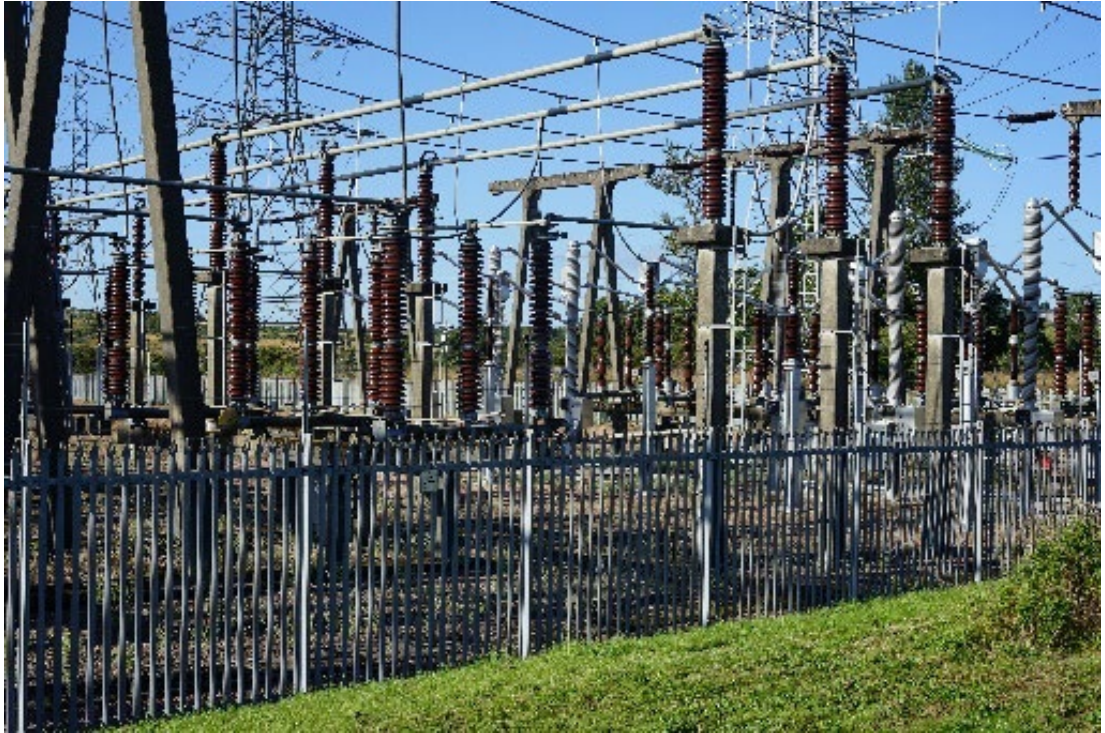
Image 3.2: Westfield Substation Existing Infrastructure.
