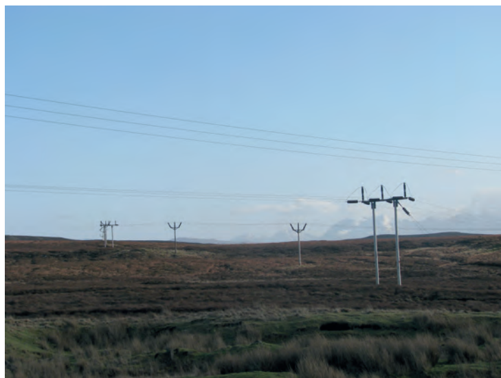
Trident single and 'H' poles in moorland setting
