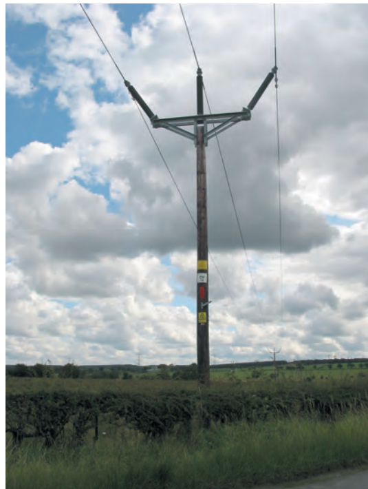
Trident single pole, 'trident' insulators
