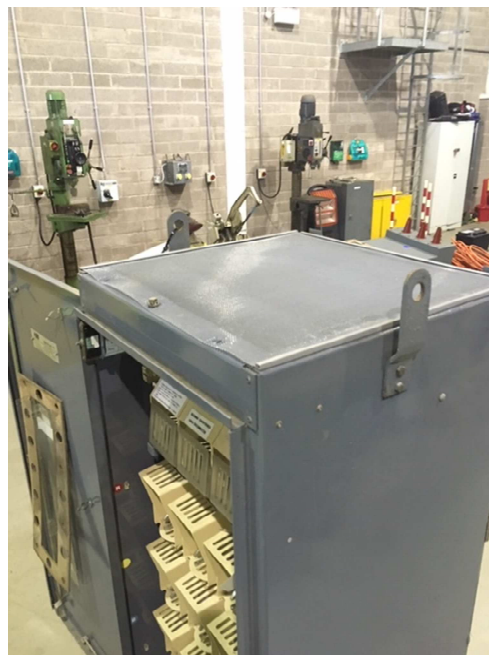
Figure 5: LV Take-Off Chamber with Wire Mesh (Lid removed)
