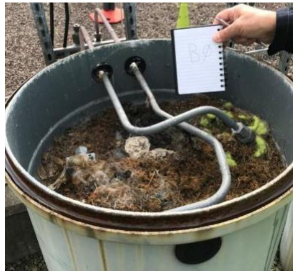
Figure 2: Fluid tank at Braehead compound showing sign of rust.
