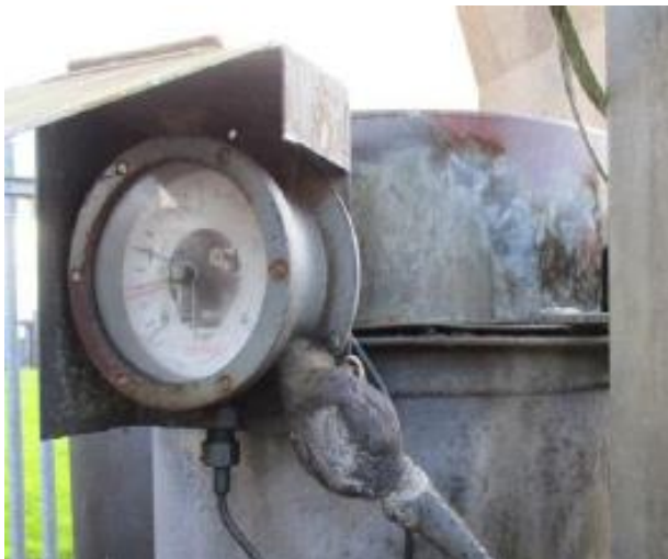
Figure 1: General condition of gauge and pipework at Red Smiddy compound.
