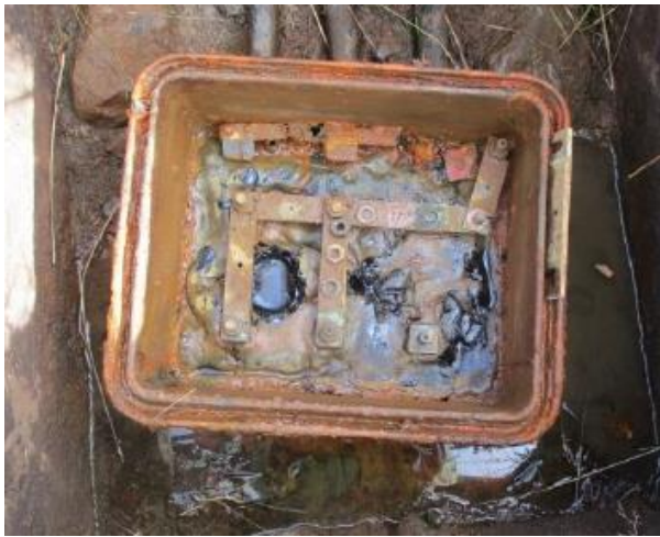
Figure 3: condition of link box at BZ15.
