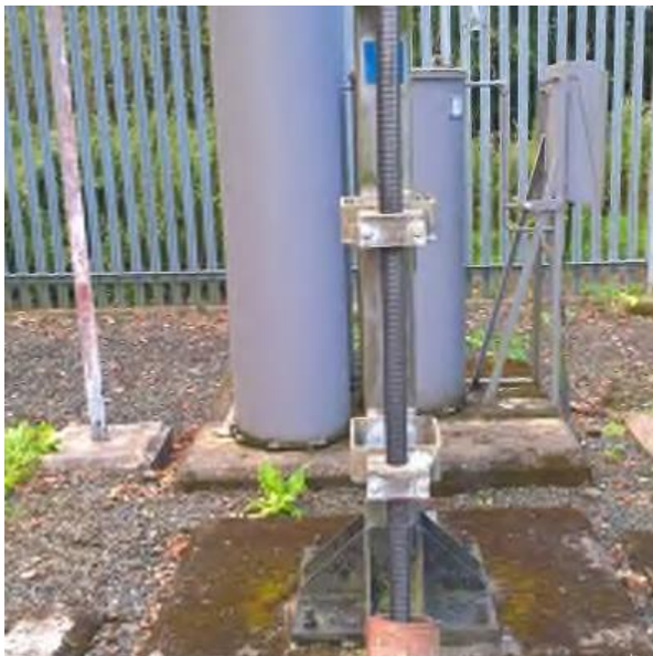
Figure 5: tanks starting to show signs of corrosion on lids and bases.
