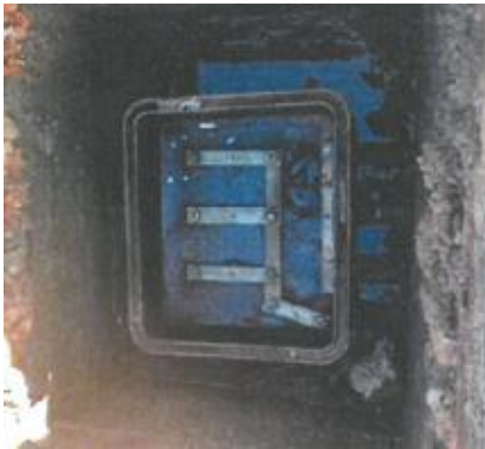
Figure 9: typical link box. Compound blistering and signs of water ingress.
