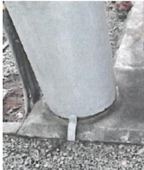
Figure 10: tanks showing signs of corrosion on bases.
