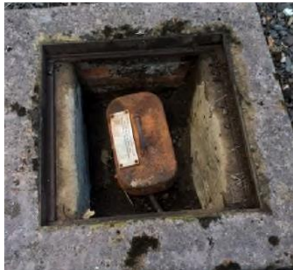
Figure 6: link box corroded.
