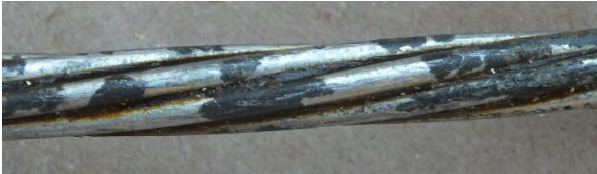
Figure 2: conductor sample showing low level of grease found between steel wires and significant loss of the galvanic zinc layer.
