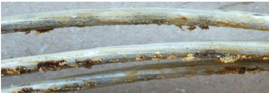
Figure 1: inner aluminium strands exhibit a significant level of aluminium corrosion product and greased discoloured and hardened.
