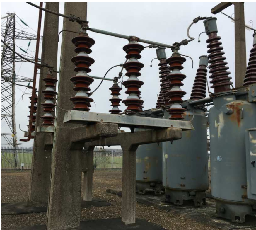
Figure 2: Existing AEI 132kV RCP Disconnector at Glenniston 132kV substation
