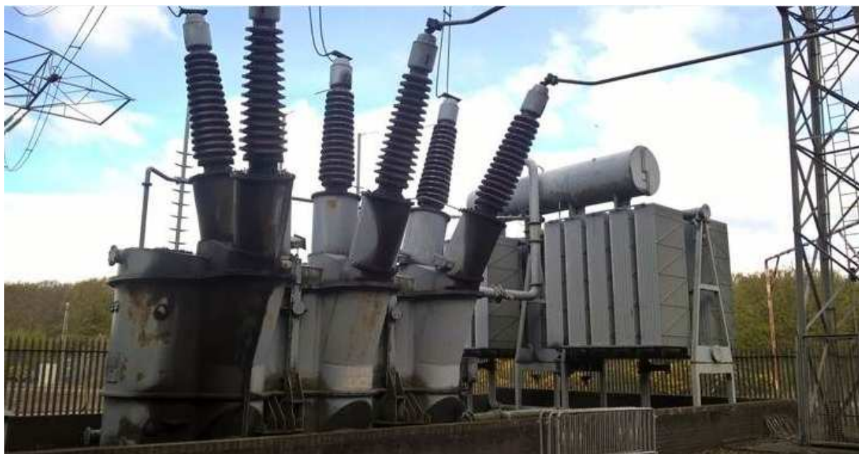
Figure 1: Longannet 275kV series reactor
